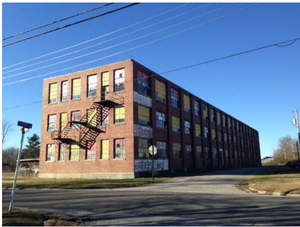
Signs of Decay: Abandoned building that has broken window panes and is boarded up.
